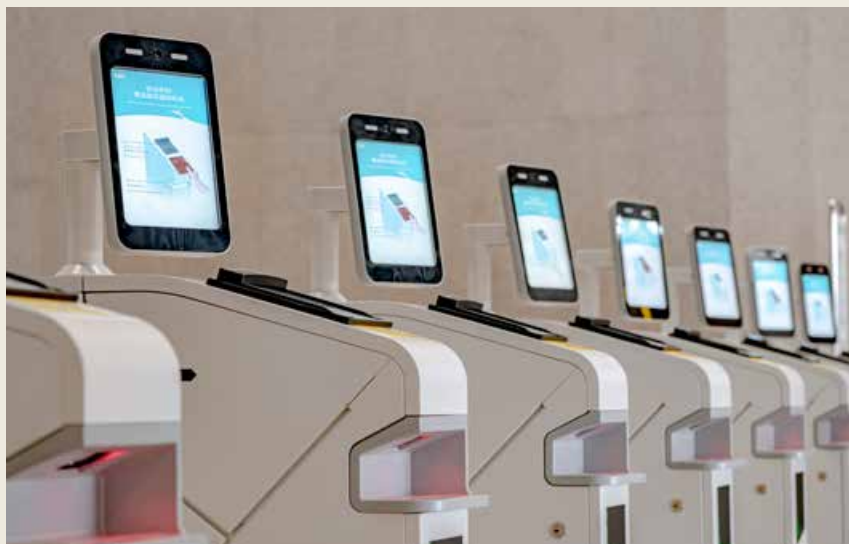
胶东国际机场通过先进的智慧机场建设，可实现自助值机、自助托运、自助安检、自助登机全流程通关。Through the advanced construction of smart airport, Qingdao Jiaodong International Airport can realize the full-process self-service facilities that comprise check-in, baggage check, security check, and boarding.
